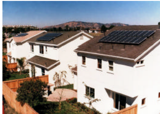
Rooftop PV system at Village Green Homes in Sylmar, CA installed by BP Solar
