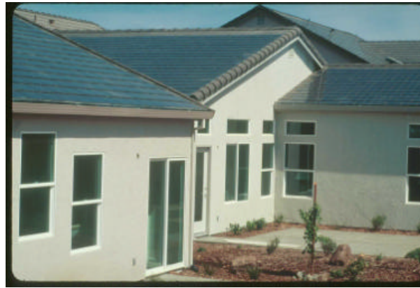
Prodigy Homes in Sacramento, CA using Atlantis Solar roof tiles under the SMUD venture
